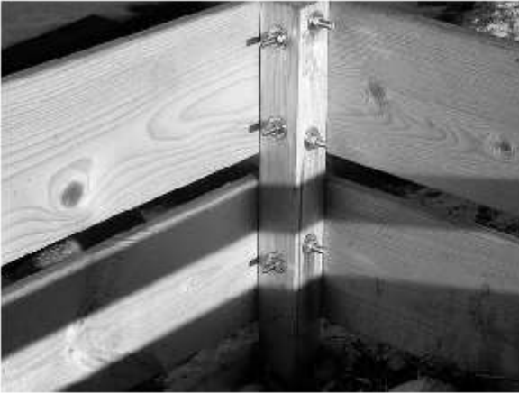
Photo 4. Detail of an inside back corner. The offset of the bolts to allow clearance through the post is quite evident. The side is on the right of the post and the back is to the left.
